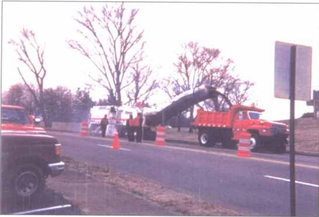
Milling to a three inch depth was done by the Tennessee D.O.T. Tuesday morning, January 11, 1994
