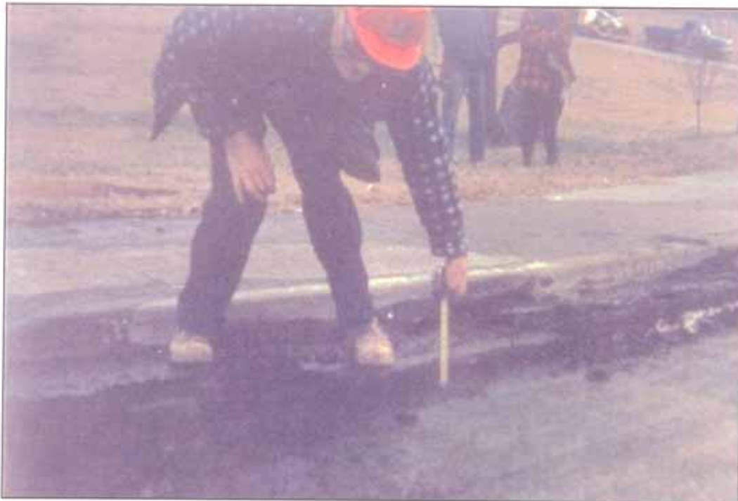
The remaining asphalt surface and gutter served as forms for the ULTRA THIN Concrete
