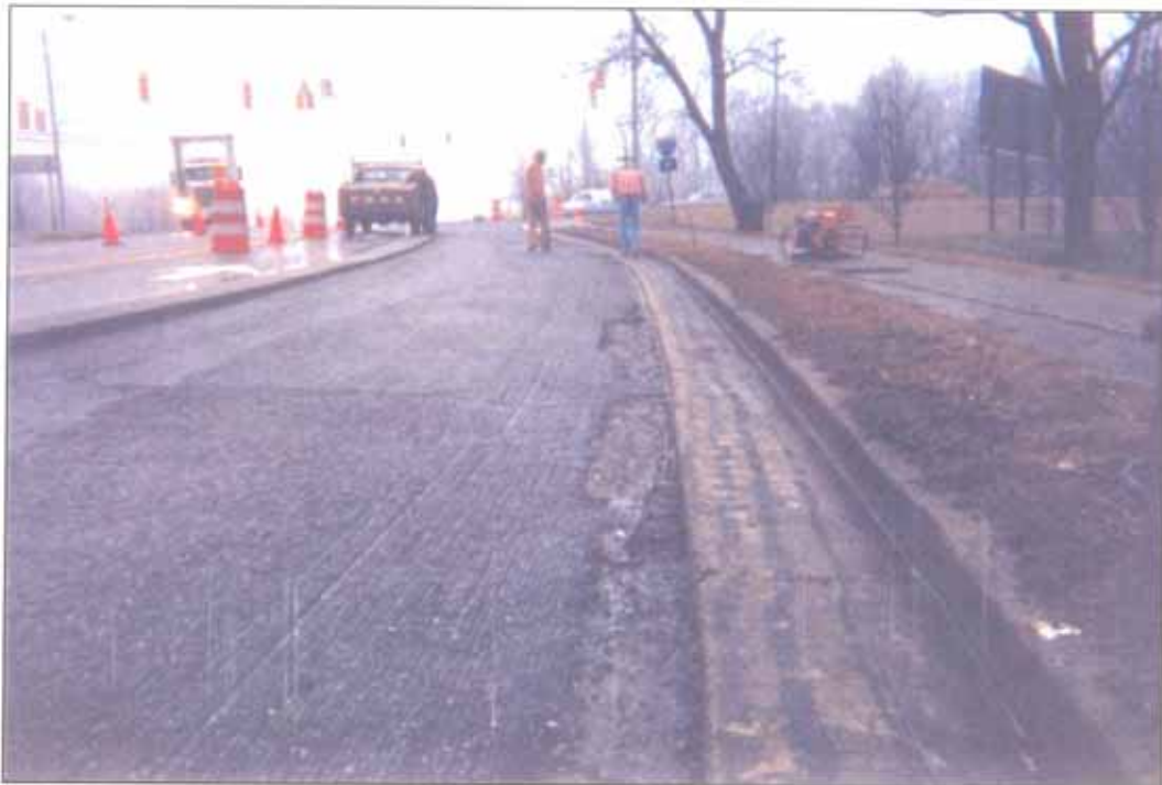
By noon Tuesday, this 188' section of road was ready for concrete Due to heavy rains in the area, concrete placing was rescheduled for Wednesday morning
